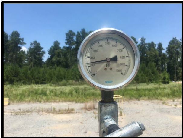
Gauge on well head
