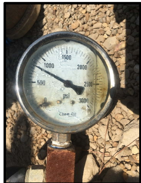
Gauge on surface casing
