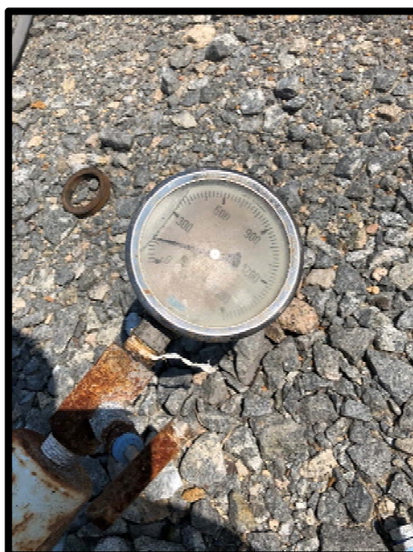
Gauge on well surface casing
