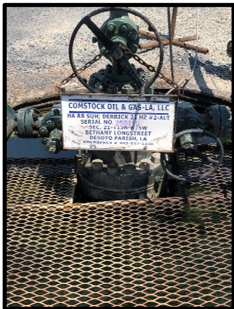
Derrick 21 HZ #2 Well Head
