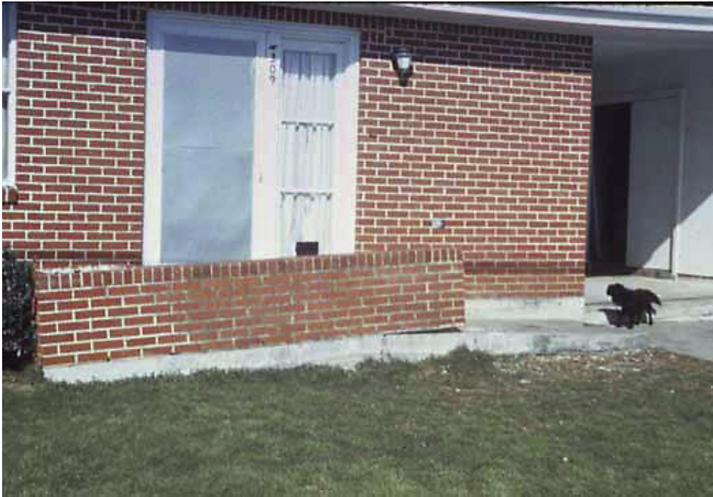
Figure 18.—Foundation failure is common for structures built on organic soils with high subsidence potential.
