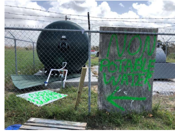
Country Pines North – LA1019083 “Non Potable Water”
