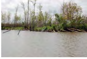
Flowlines S Schooner E Facility 116
