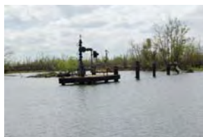
Well S Schooner E Facility 117
