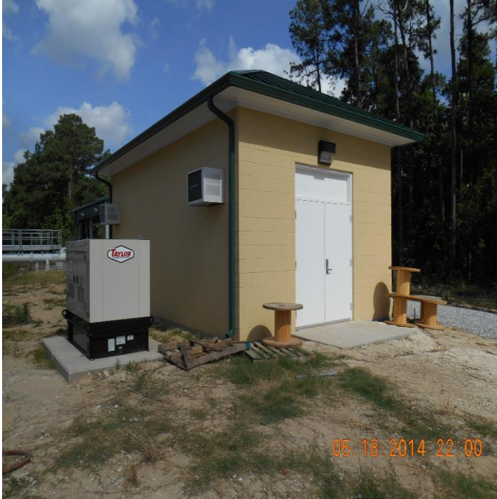
Control Building & Generator
