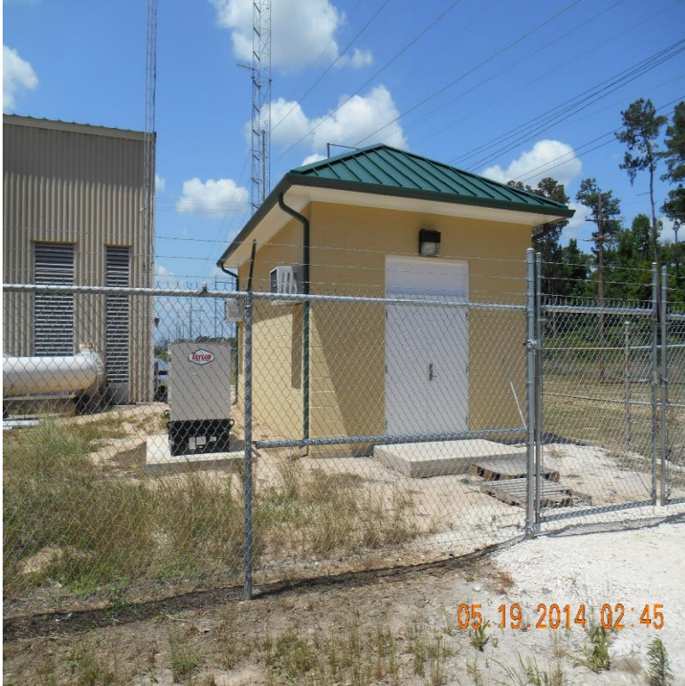
Control Building and Generator
