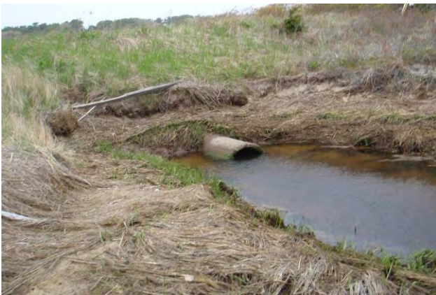
Flow Restriction - Culverts
