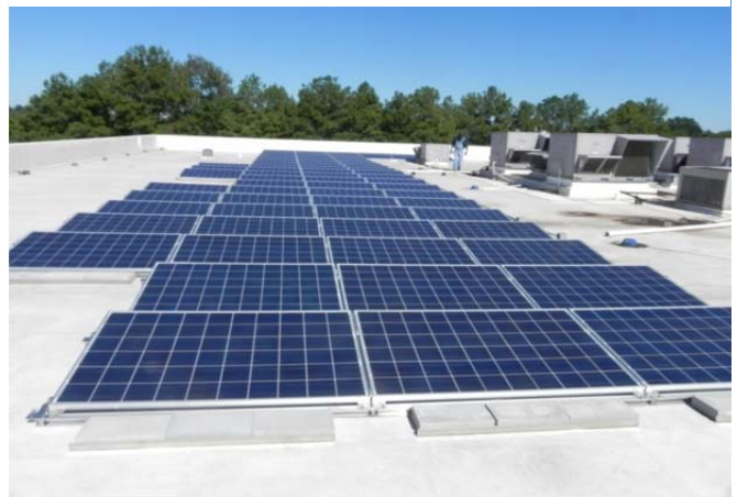
Figure 2. Solar Photovoltaic System on Webster Parish Police Jury Annex
