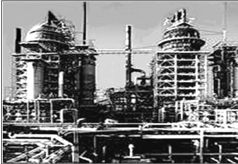
Exxon-Mobil Refinery - Baton Rouge
