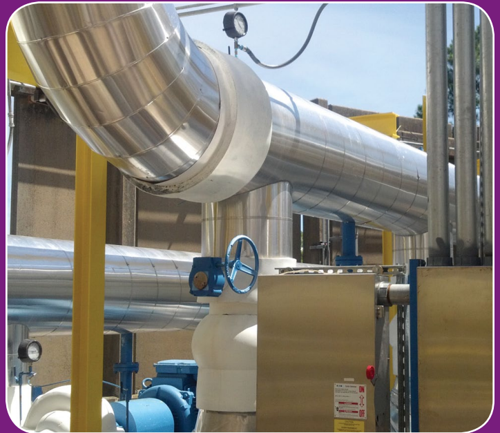
UNIVERSITY OF NEW ORLEANS STATE BUILDINGS - LEAD BY EXAMPLE HVAC
