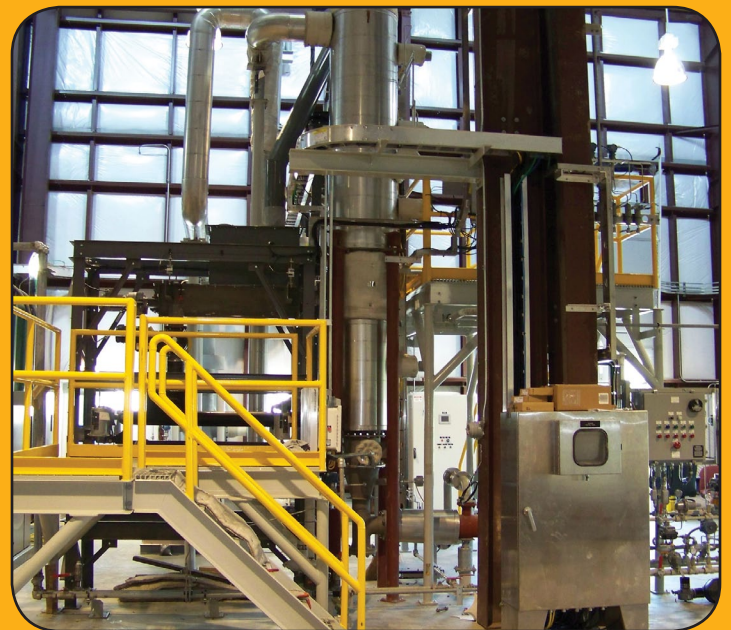
CLECO POWER LLC RENEWABLE ENERGY PROGRAM BIOMASS GASIFIER PROJECT
