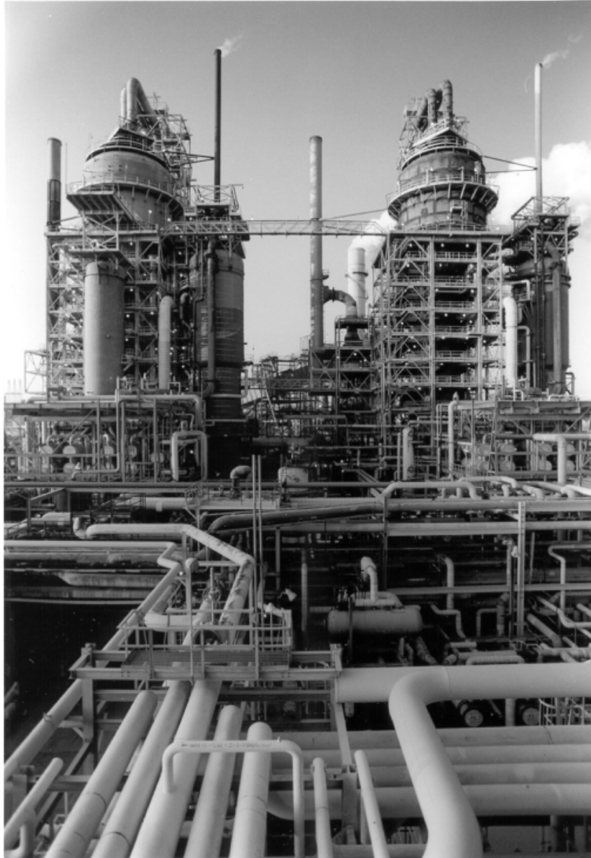
Catalytic cracking technology invented at Exxon Baton Rouge in 1942 helped win WWII. It remains industry standard. Photo courtesy Exxon Public Affair
