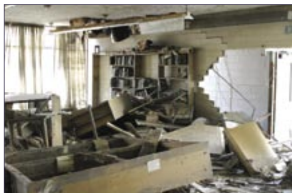
Damaged wall and furnishings in the library of the Alfred Lawless School, May 2006.
