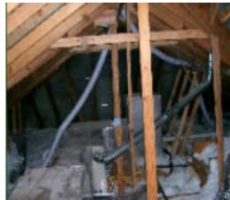
Figure 5-10. HVAC unit in attic.
