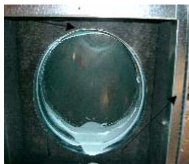
Figure 9-19. Source of leaks in register.
