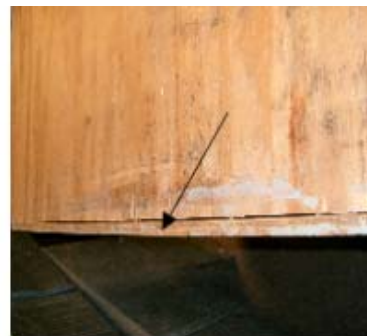
Figure 9-2. Gap along the edge.
