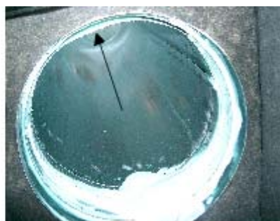
Figure 9-18. Leakage spot after applying sealant
