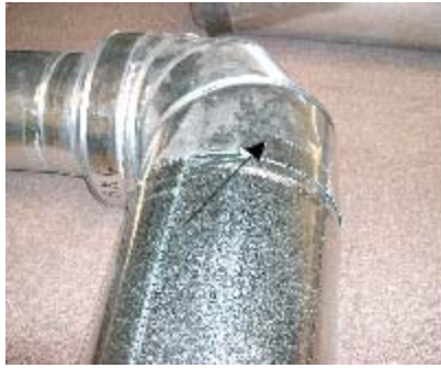
Figure 9-11. Seam of the duct system.
