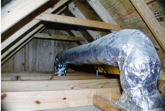
View of the attic in the non-insulated bldg. (Only the simulated duct system in the non-insulated bldg. was Insulated)
