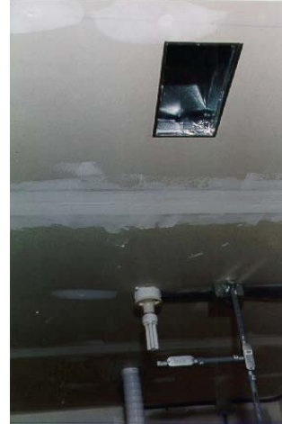
Air was circulated through a duct to simulate duct pressure and prevent air stratification
