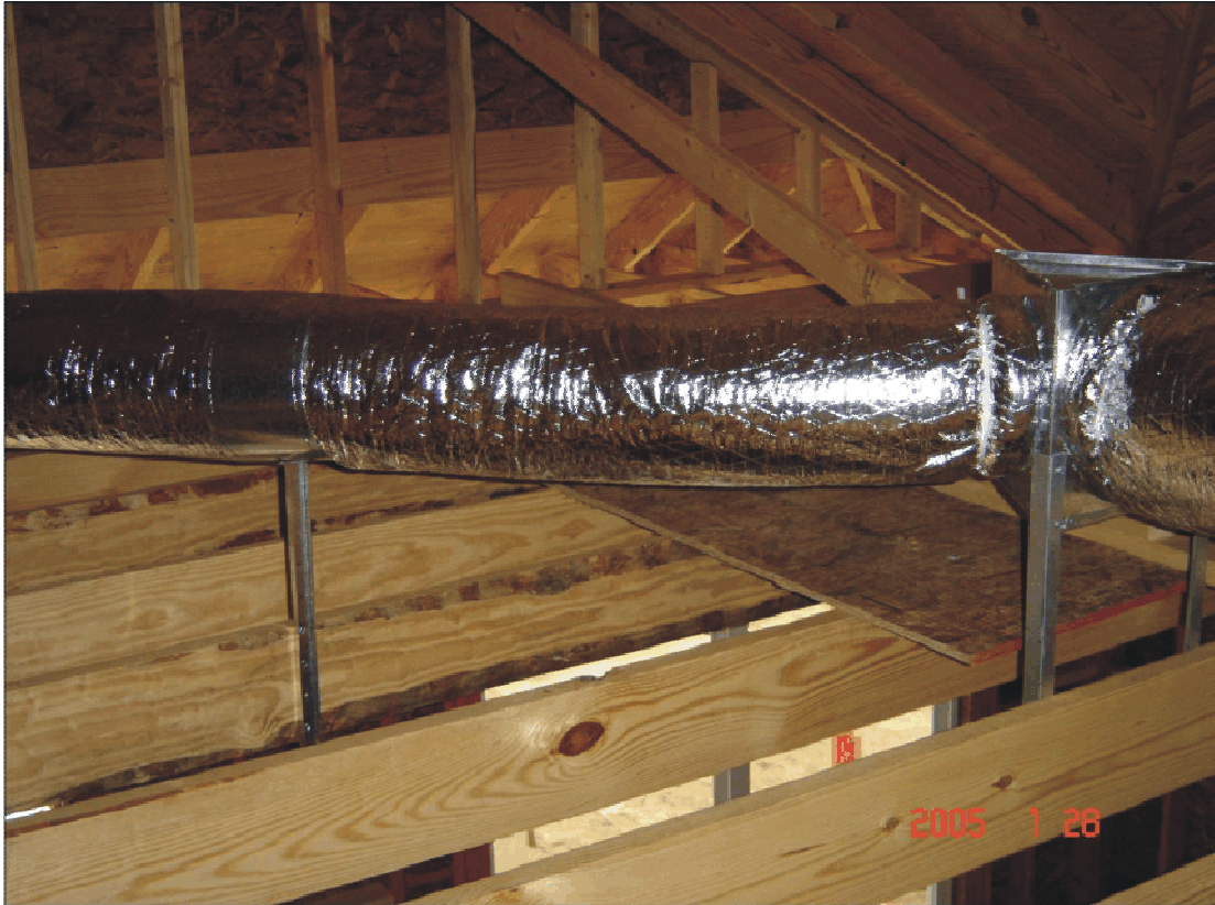
Example of a good flex duct installation (straight, fully extended, properly secured, and sealed with mastic)
