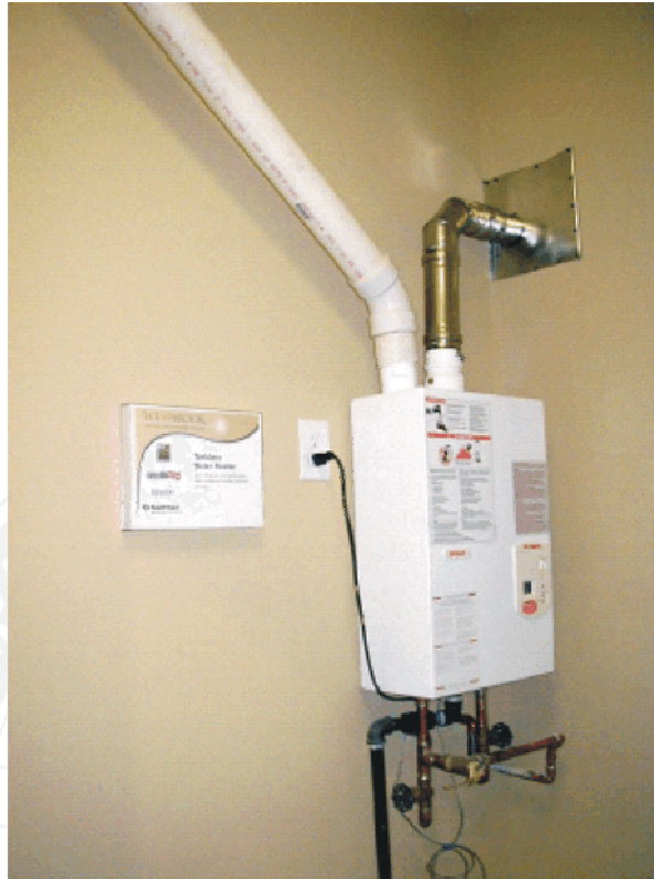
Large capacity gas instantaneous water heater (note that the circuitry for the instantaneous water is basic wall power – low current)
