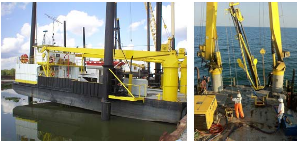
Figure 6 - Photographs of EBI® liftboat. Right photo shows OSI crew recovering a core utilizing one of the stern-mounted cranes permanently installed on the vessel.
