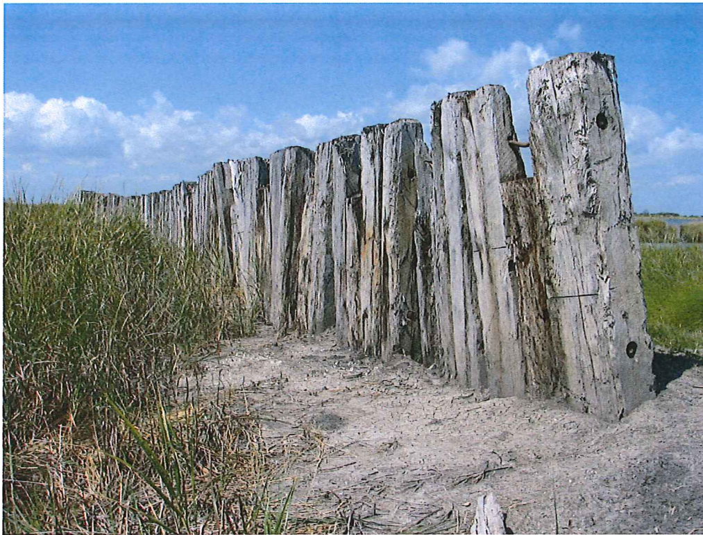
Figure 1. Bid Item 4 - Timber Mats (Date Taken 9-26-12)
